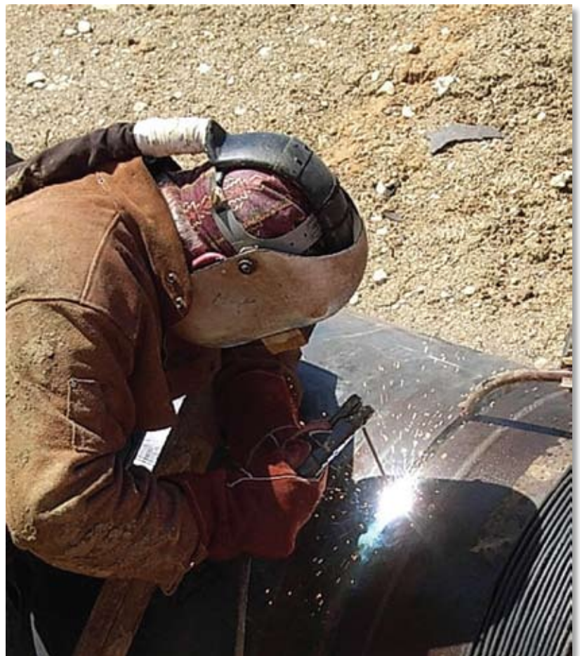
Fig. 1. Arc blow problems can causing severe project delays.
