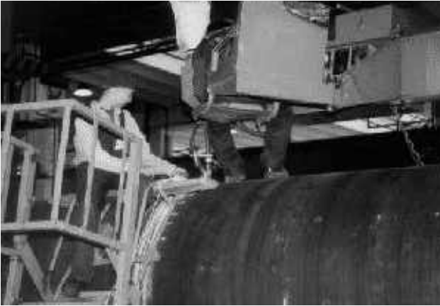
Fig 4. Welding of a circumferential joint being carried out while demagnetisation is in process
