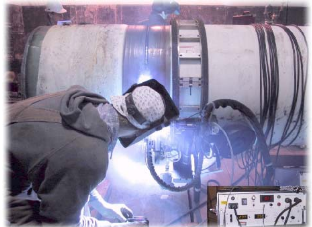
Fig. 1. Zeromag in use on underground pipeline
