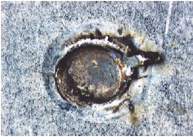
Surface splash and surface cracking in coated steel
